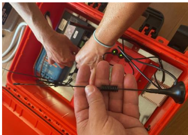
Figure 27. Antenna installed in LOPI1, LOPI2, LOPI3 and LOPI4 stations.
