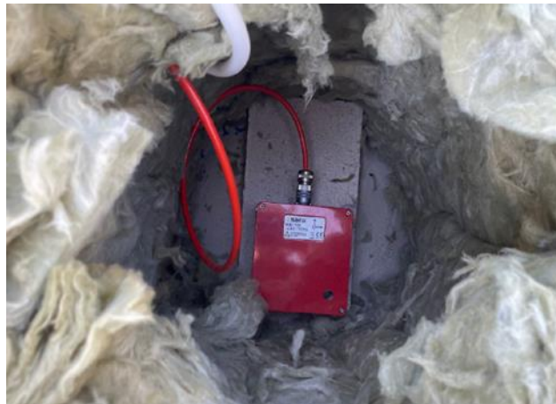
Figure 24. Seismic sensor, leveled and north oriented
